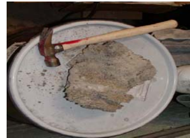
Large clinker from burner box.
