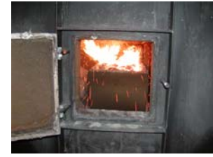
Pellet burner box.
