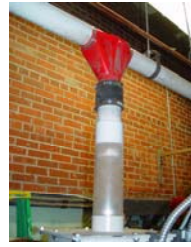
Feed tube dropping pellets into burner.
