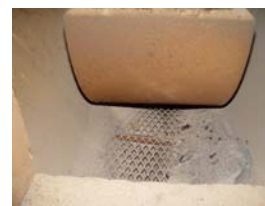
Screen installed to catch clinkers.
