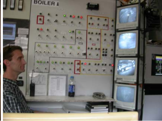
Portion of boiler Monitor panel
