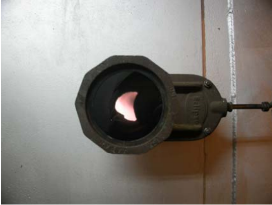
Upper fire chamber viewing port
