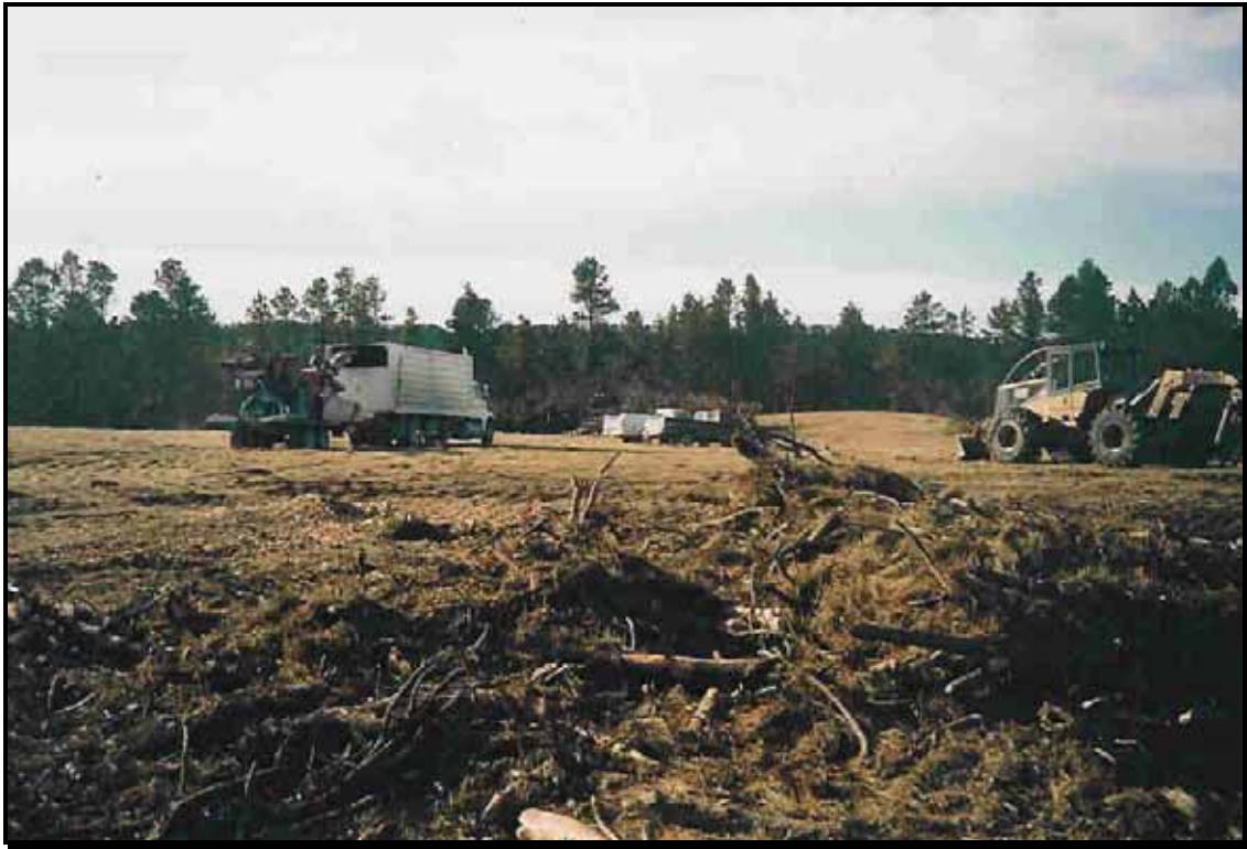
Photo 13: Moving the chipper to the next pile. Pile estimated to contain 20 truckloads of chips.
